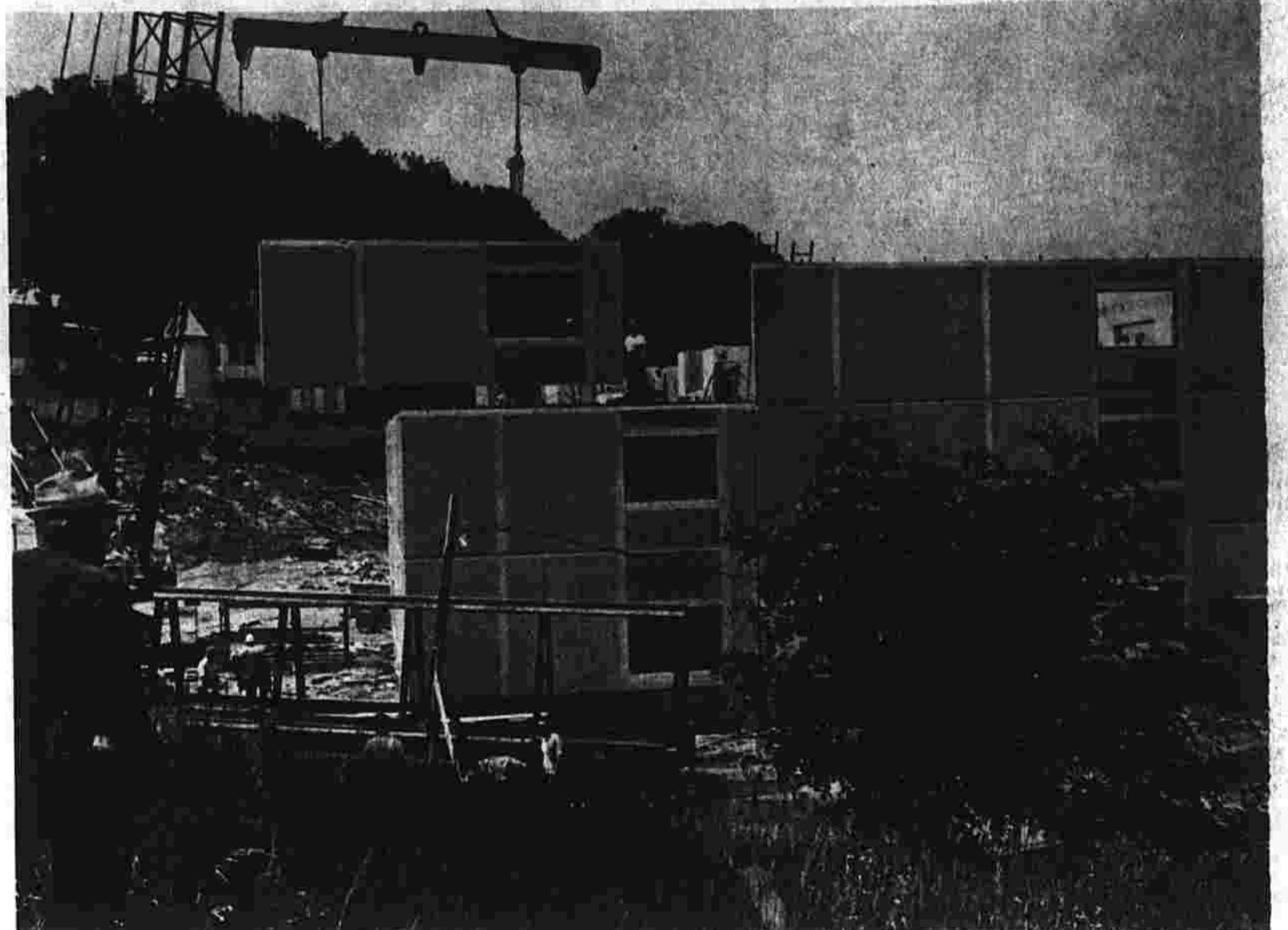
Third Floor—Going Up Workers at the redevelopment site in Rockville guide into place one of the 11-ton prefabricated panels of the six-story highrise apartment complex for the elderly. Lifting the panel is an 85-ton crane. The building is being constructed by C. W. Blakeslee Corp. of Branford for Alco Development Corp., developers of the renewal area. When completed, the building will be turned over to the Vernon Housing Authority. It will be the town's fourth elderly housing project. (Herald photo by Buccivicus)
